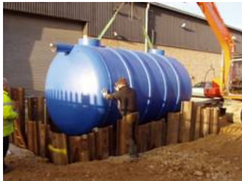
New Rainwater Harvesting Tank
